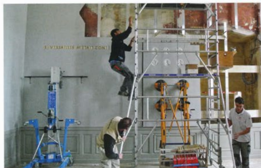
Figure 4 – A system of aluminum frames were affixed to the palace walls to hold the panels in place.
